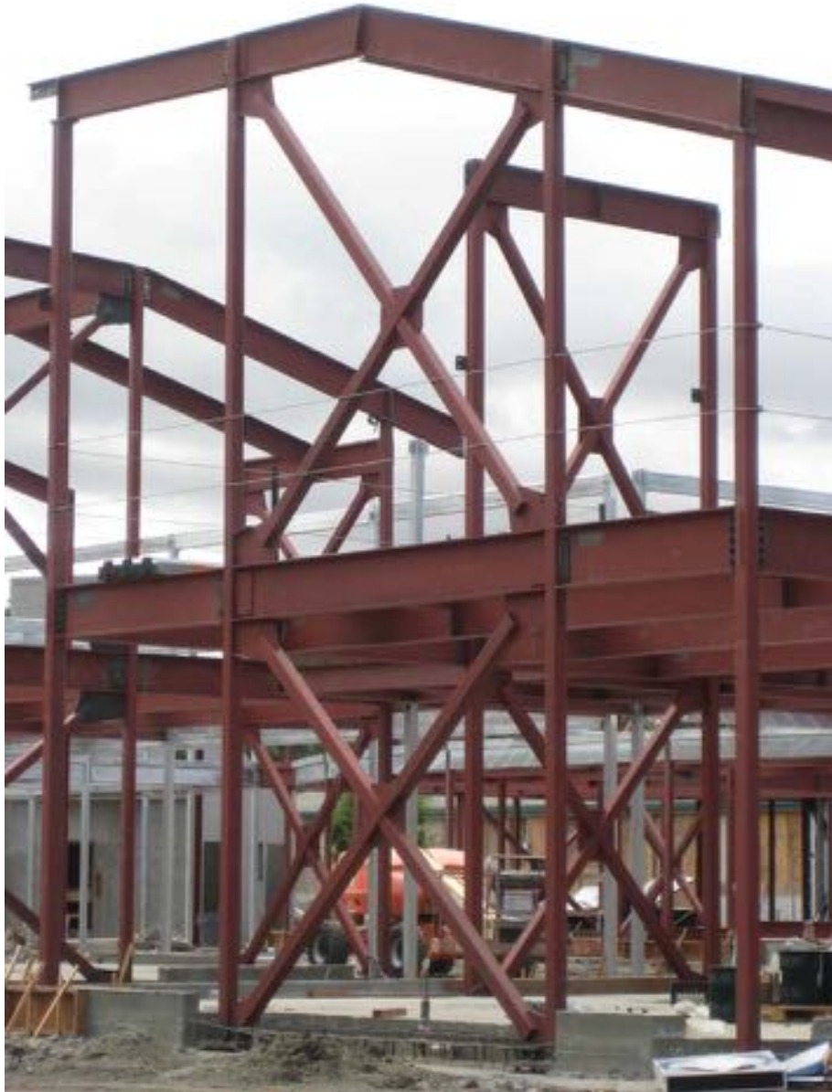
Figure 19: The triangular members in the model act the same as the larger shear bracing seen here on this school under construction, Menlo Park CA. Notice that not every wall has the shear supports, hence the thicker shear braces.
